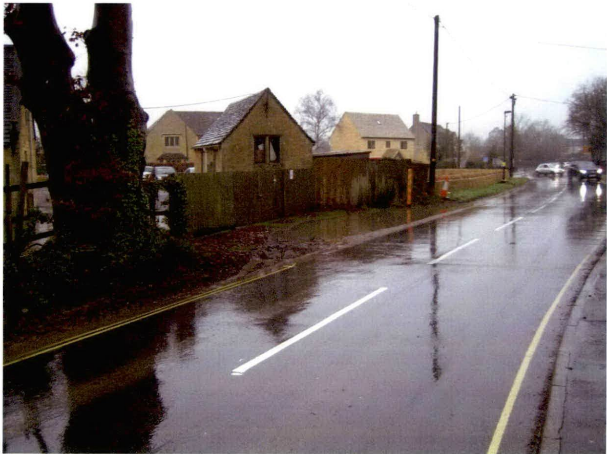
Area of Flooding due to damaged/affected Soakaways & Highway Gullies.
